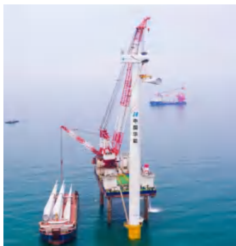
Offshore Wind Tower China Huaneng Group CZ1 Offshore Wind Farm Project, Lingao County, Hainan MySE10-242 10MW
