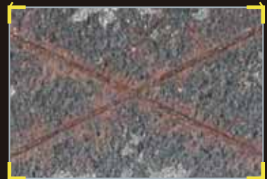
Rust is found other than cross-cut.
