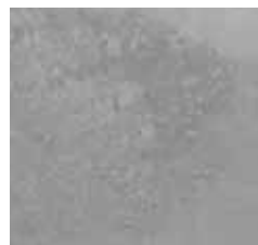
After 6 months exposure
