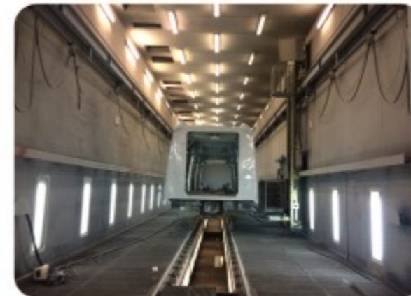
Railway Locomotive shotblasting Booth
