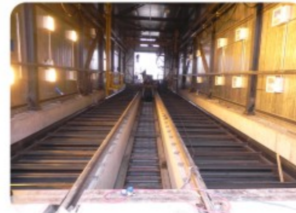
Scrap Recovery shotblasting Booth
