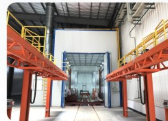
Rail Vehicle Paint Booth
