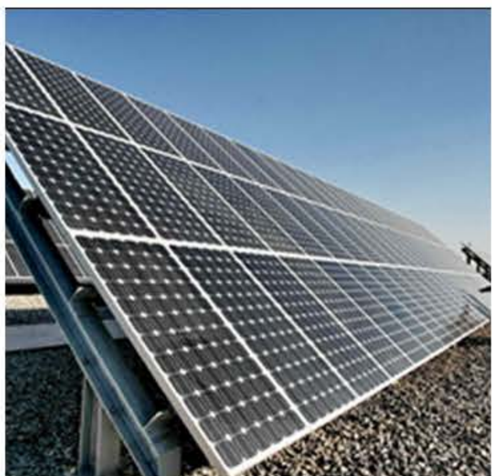
光伏发电 PHOTOVOLTAIC GENERATION
